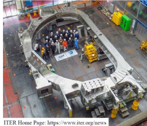
Fig. 1 The first assembly of TF coil case. The joints of in-board and out-board coil cases locate at the top and the bottom of the coil structure.
